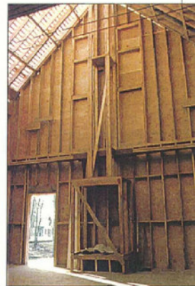
Reinforcing with plywood and steel. In the absence of collar ties, 1-in. dia. steel tie rods supported by angled stays keep the tall walls from spreading. Because the rafters are skip-sheathed to allow the cedar roof to breathe, adding another layer of ½-in. plywood on the interior of the framing helps to stiffen the roof and walls against the wind.
